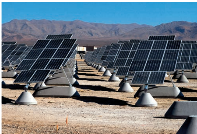
figure 1.9 A power plant at Nellis Air Force Base utilizes photovoltaic solar cells.
